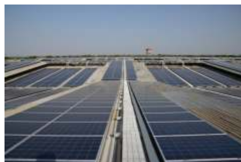
Adanis set up ₹ 315 - crore Solar PV Plant in UP
